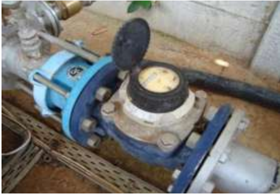
Flowmeter not functional at boreholes
