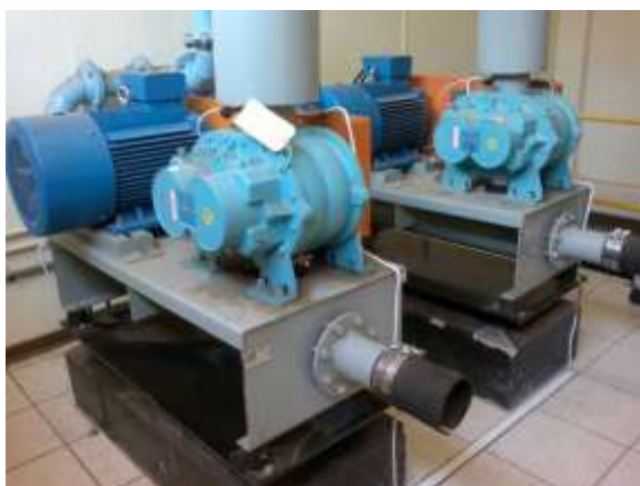
Two blowers are available – one operational, one standby
