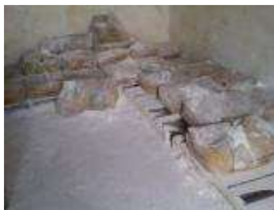
Poor housekeeping in the lime storage area
