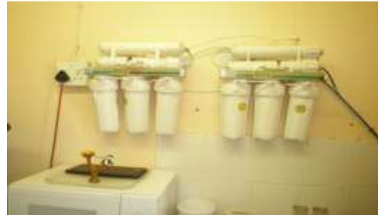
A filtration system is used to remove fluoride from the water
