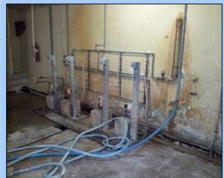
Chemical dosing facility at Witbank WTW requires housekeeping.
