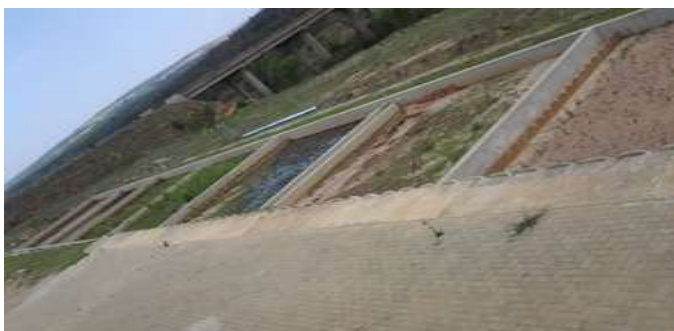
The sludge dams not well maintained (grass growing)
