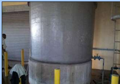
Chemical storage area lacking bunded
