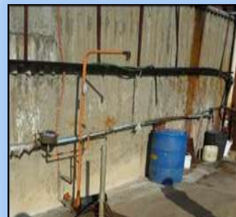
Emergency shower and eyewash in need of routine service
