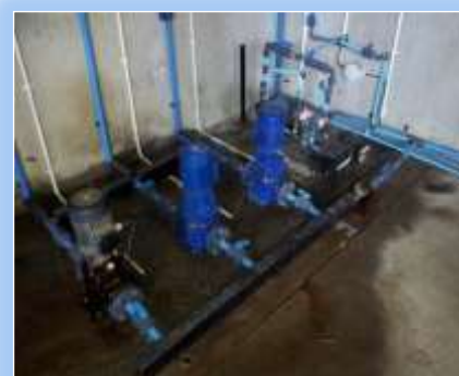
Chemical dosing room with 2 dosing pumps not working and loose electrical wires.
