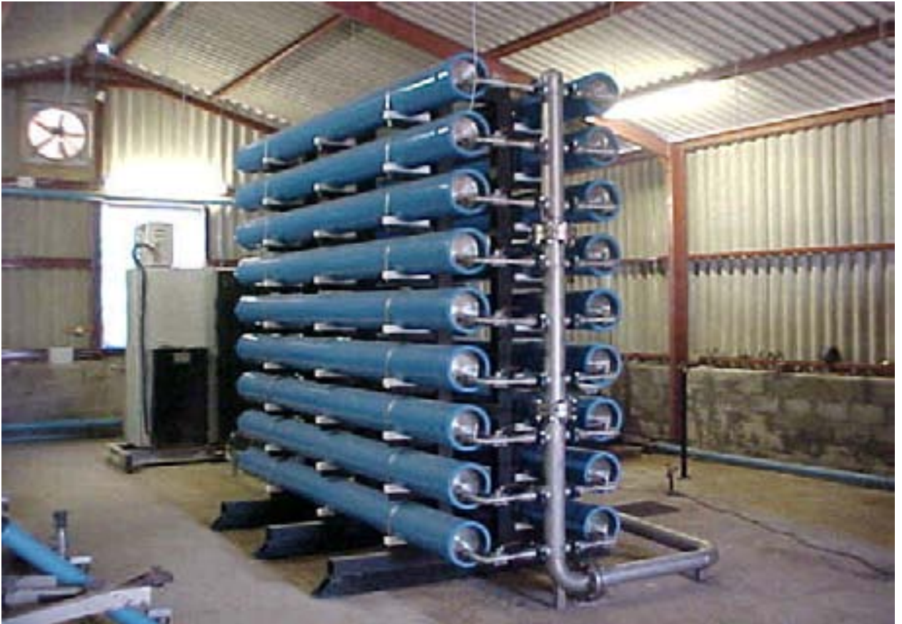
Plate 17: RO Plant at Kenton on Sea
