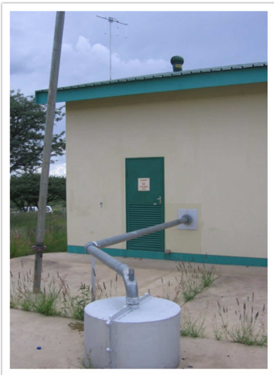
Photo 5: One of Windhoek's injection boreholes
