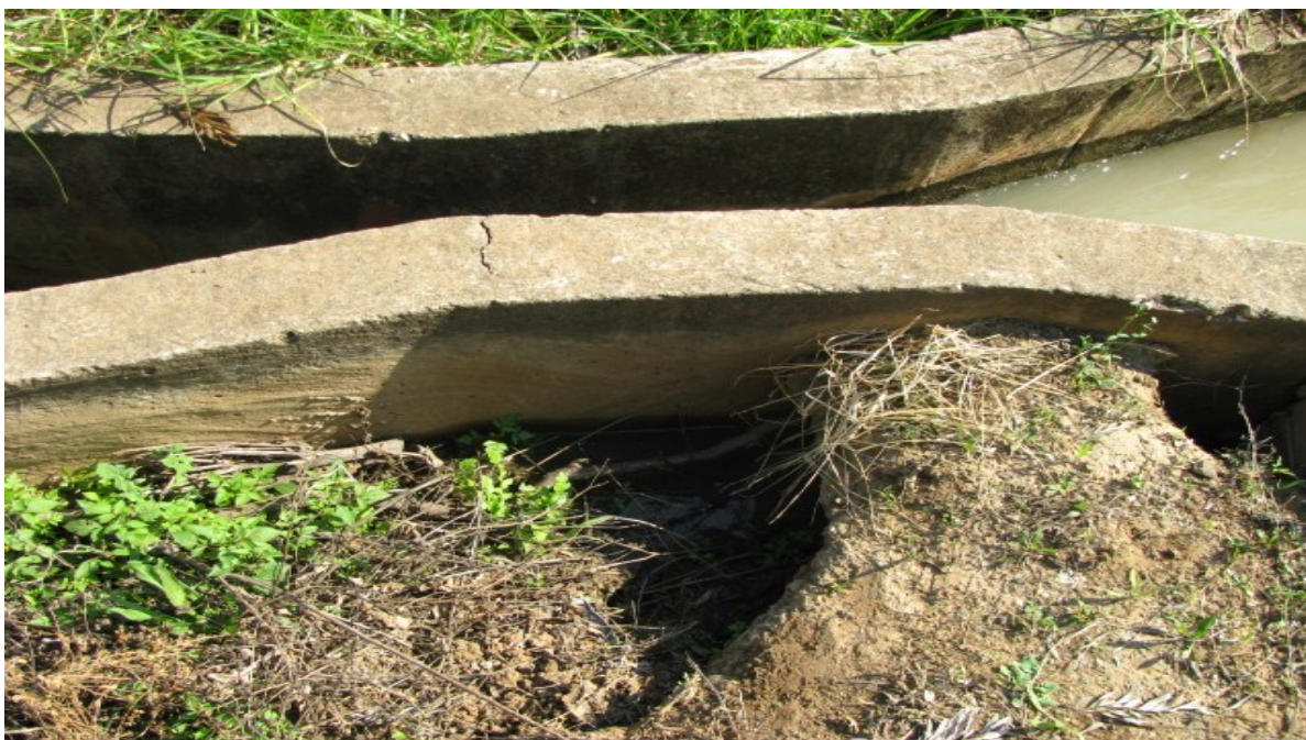
Photo 5.3: Erosion around the sides of a branch canal
