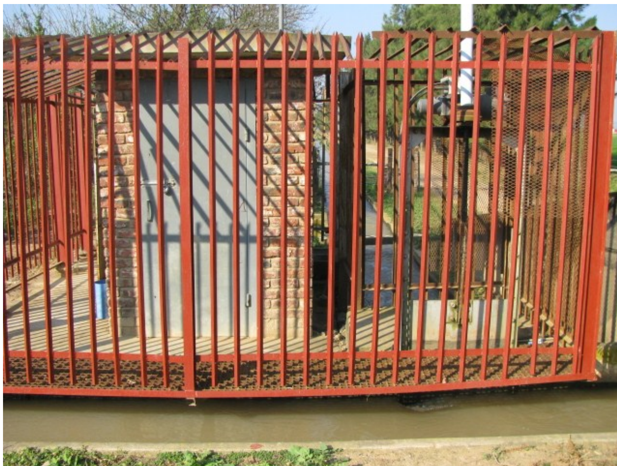
Photo 5:6: Remote Telemetry Outstation (RTU) on the Kirkwood primary canal which was not operational
