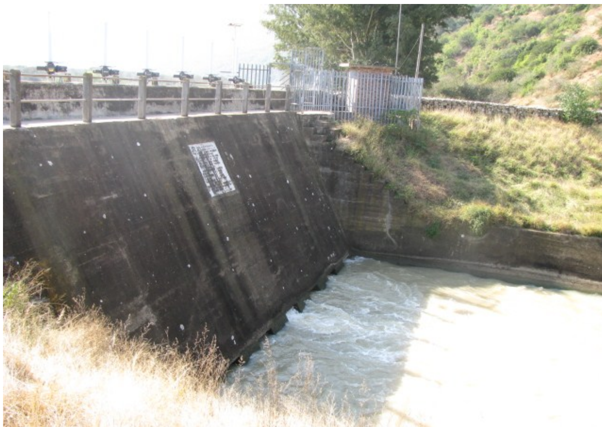
Photo 4:2: View of the inlet into the main canal with the automated rotork valves and remote telemetry unit (RTU)
