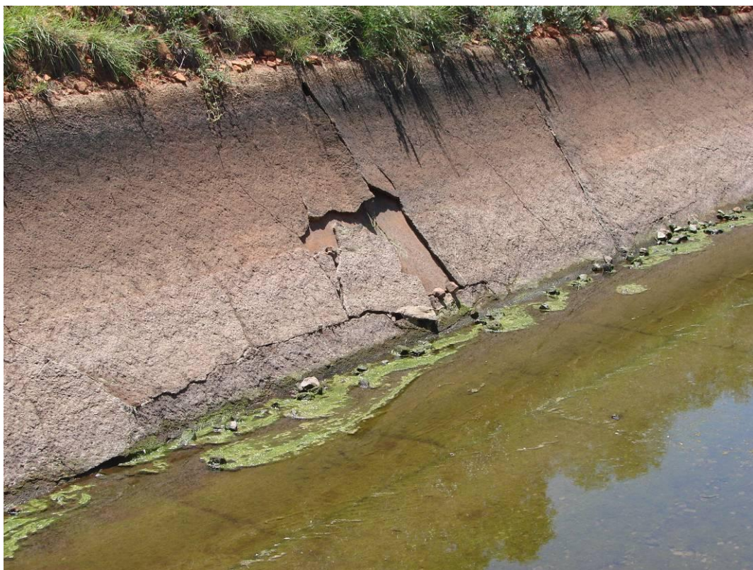
Figure 4-1 Deteriorating canal structure (left bank)
