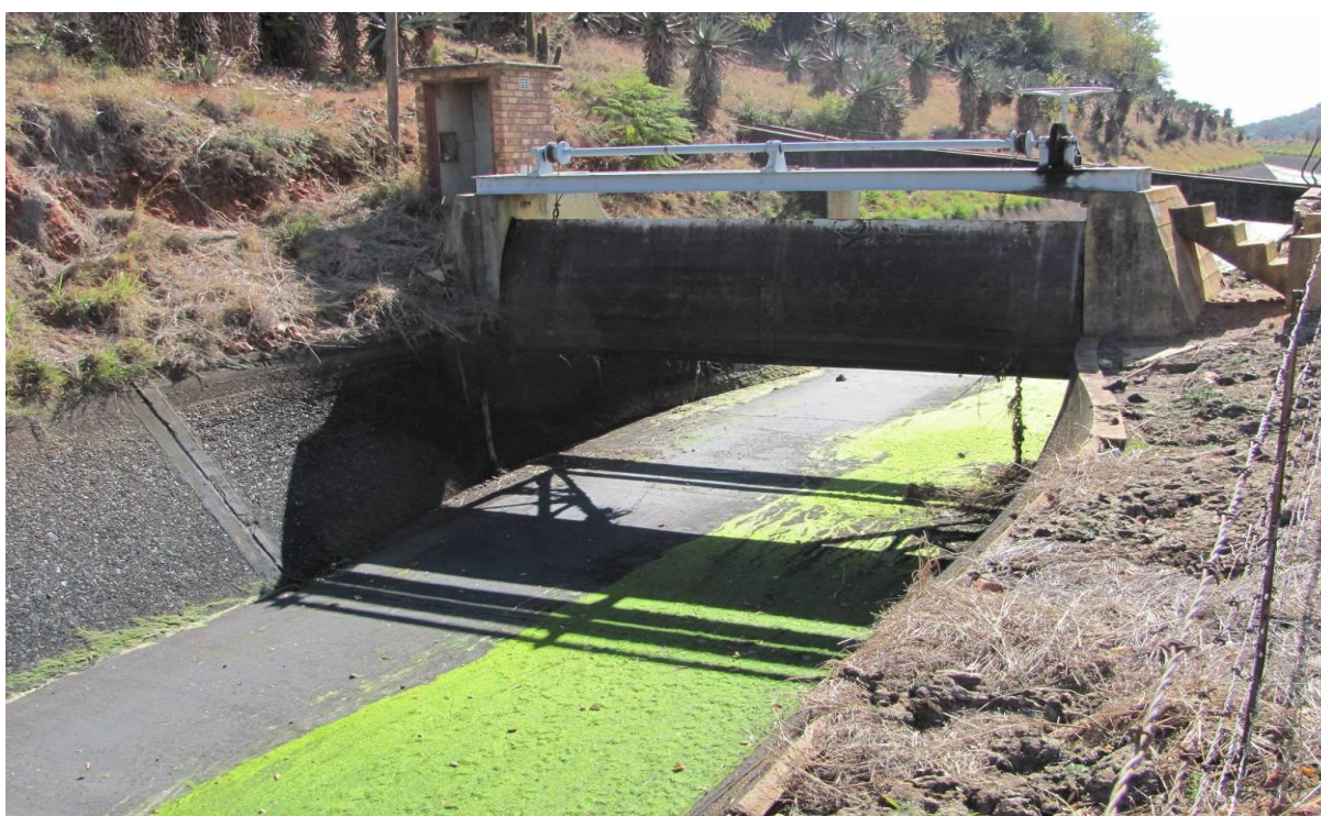
Figure 7-4: Algae growth in the canal system and radial gate
