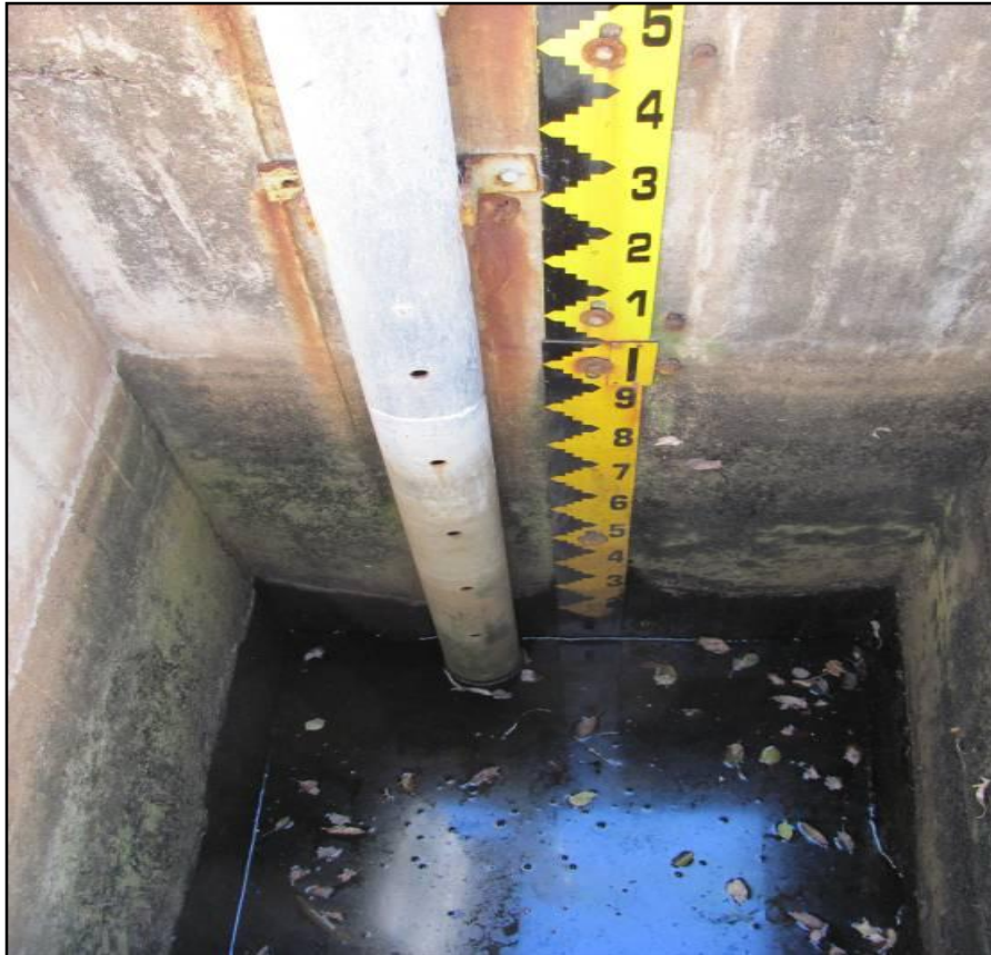
Photo 3-2: Telemetry system at the left outlet of Loskop Dam
