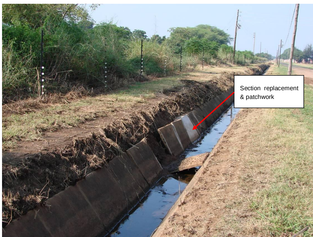
Figure 4-4 Canal failure and refurbishment (right bank)
