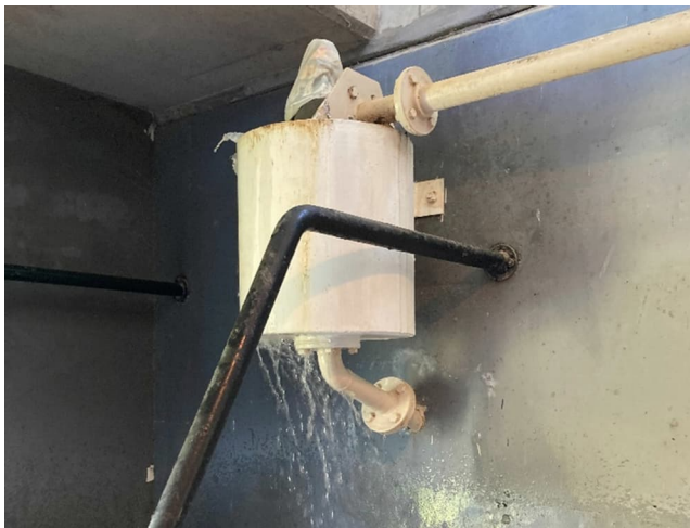
Figure 3-61: Filter float chamber overflowing
