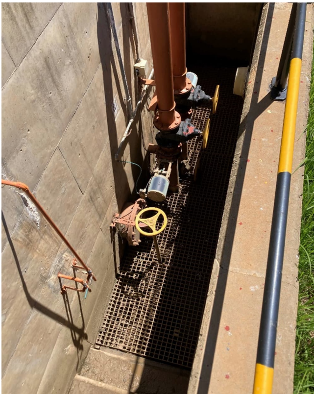
Figure 3-57: Pulsator de-sludge valves (actuators not operable)
