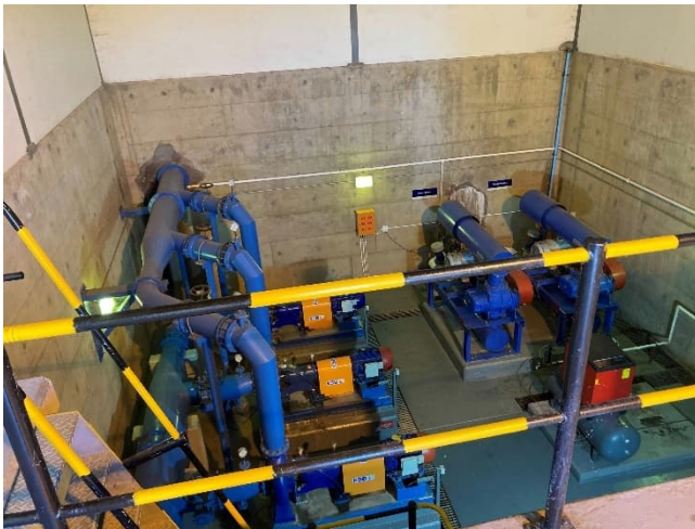
Figure 3-63: Filter backwash pumps and air scour blowers
