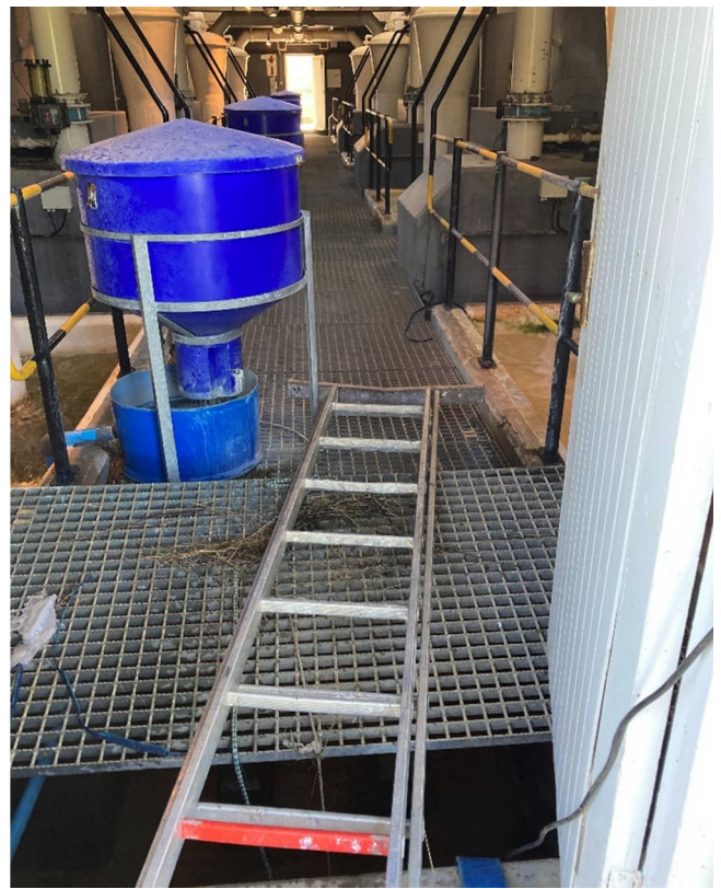
Figure 3-60: Lower filter gallery (unsafe access)
