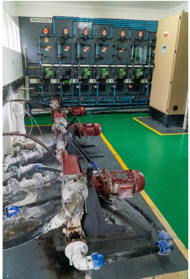
Figure 3-38: Lime slurry dosing pumps
