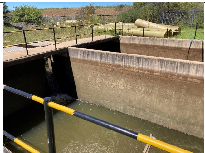
Figure 3-66: Residuals holding tanks
