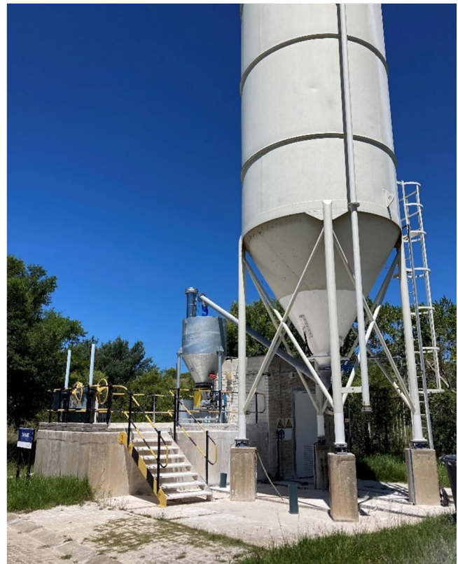
Figure 3-50: Lime dosing equipment
