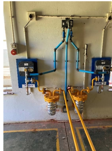
Figure 3-64: Chlorine dosing equipment
