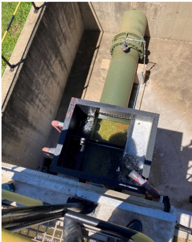
Figure 3-49: Inlet chemical dosing and flow splitting
