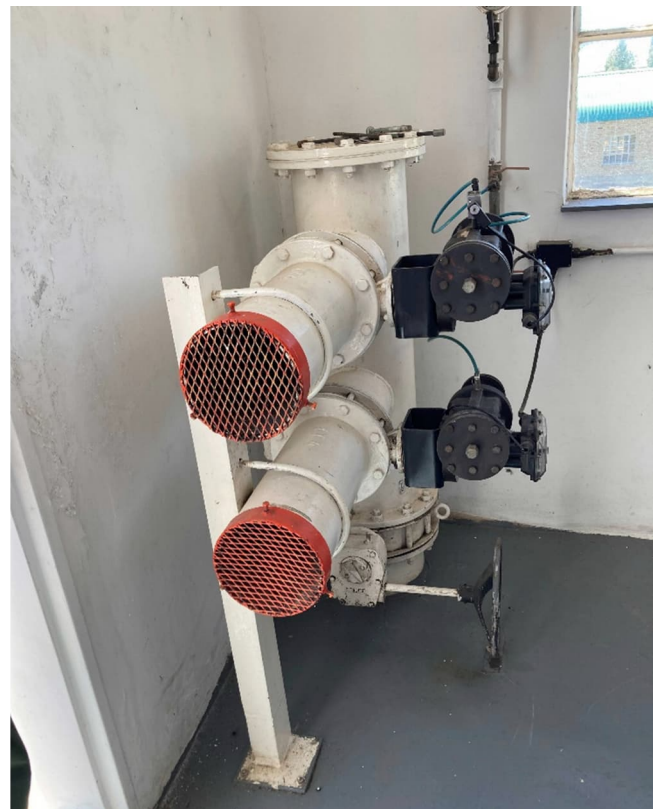
Figure 3-56: Pulsator vacuum control equipment (not operable)
