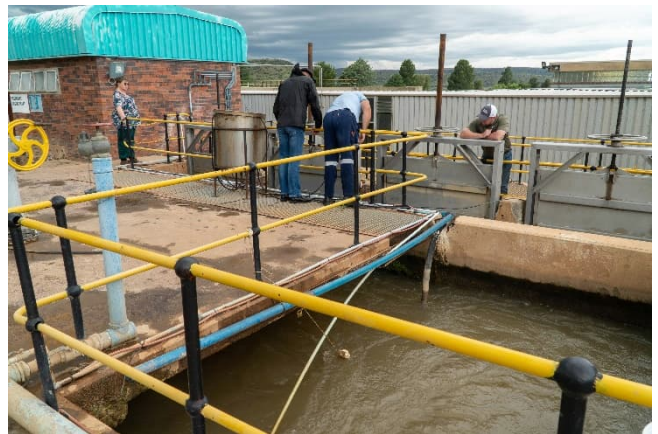
Figure 3-42: Agitators and secondary dosing point
