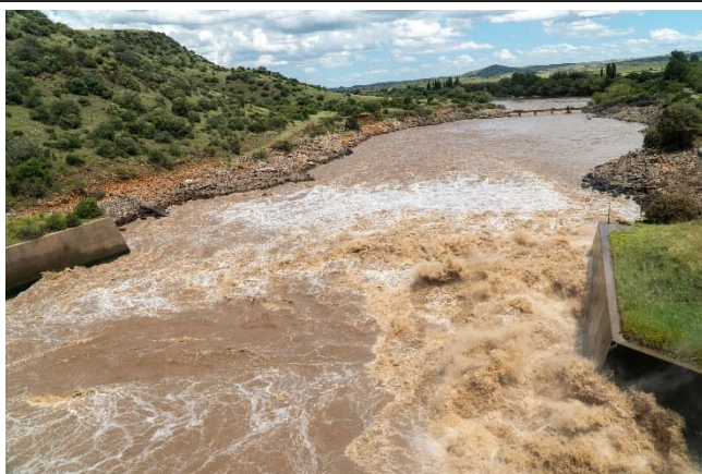
Figure 3-33: Evidence of downstream scouring and debris
