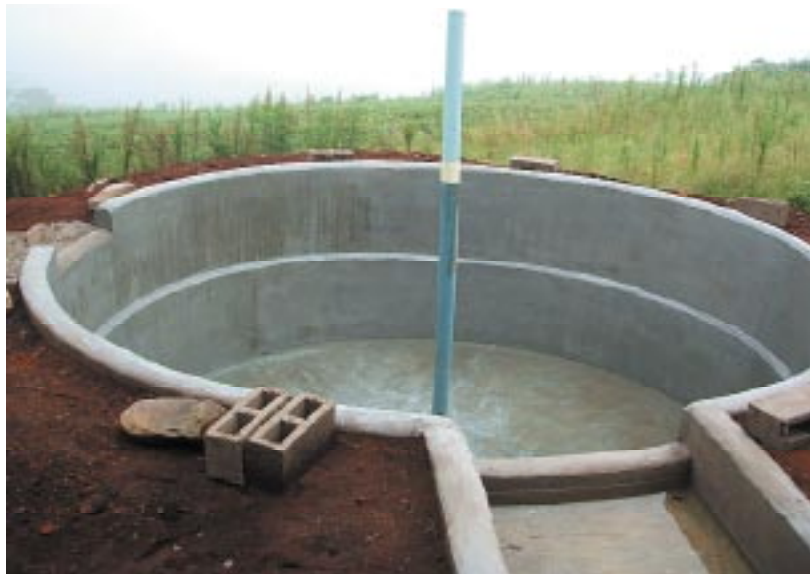
Figure 3: Typical 30 m 3 rainwater tank
