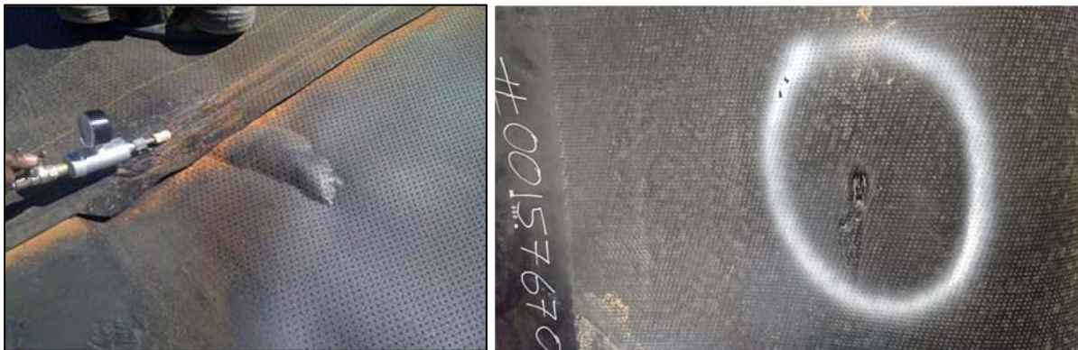
Figure 1: Geomembranes manufactured to ISO 9001 but shipped and revealed deviations from performance during construction (a) Separation in plane adjacent to wedge welds and (b) Discontinuities in texturing and thickness to the extent of manufactured holes.
