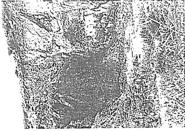
PLATE 12 - Note failure at the crest of the slope and loose scree at the toe of the slope.
