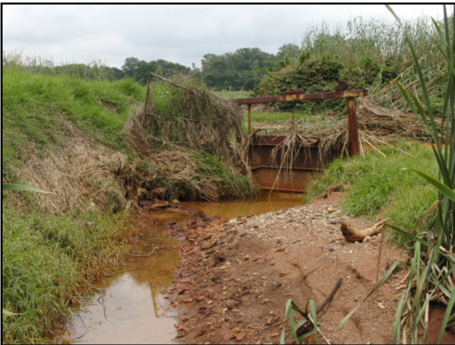
Plate 2. View from downstream of the sluice gate at the entrance to the A-furrow downstream of the Zwartkrans Spring following the high discharge conditions experienced in the Bloubank Spruit in mid-December 2010; note the disruption of flow into the furrow and the sediment deposition on the left bank (right foreground). (Photo: Phil Hobbs).
