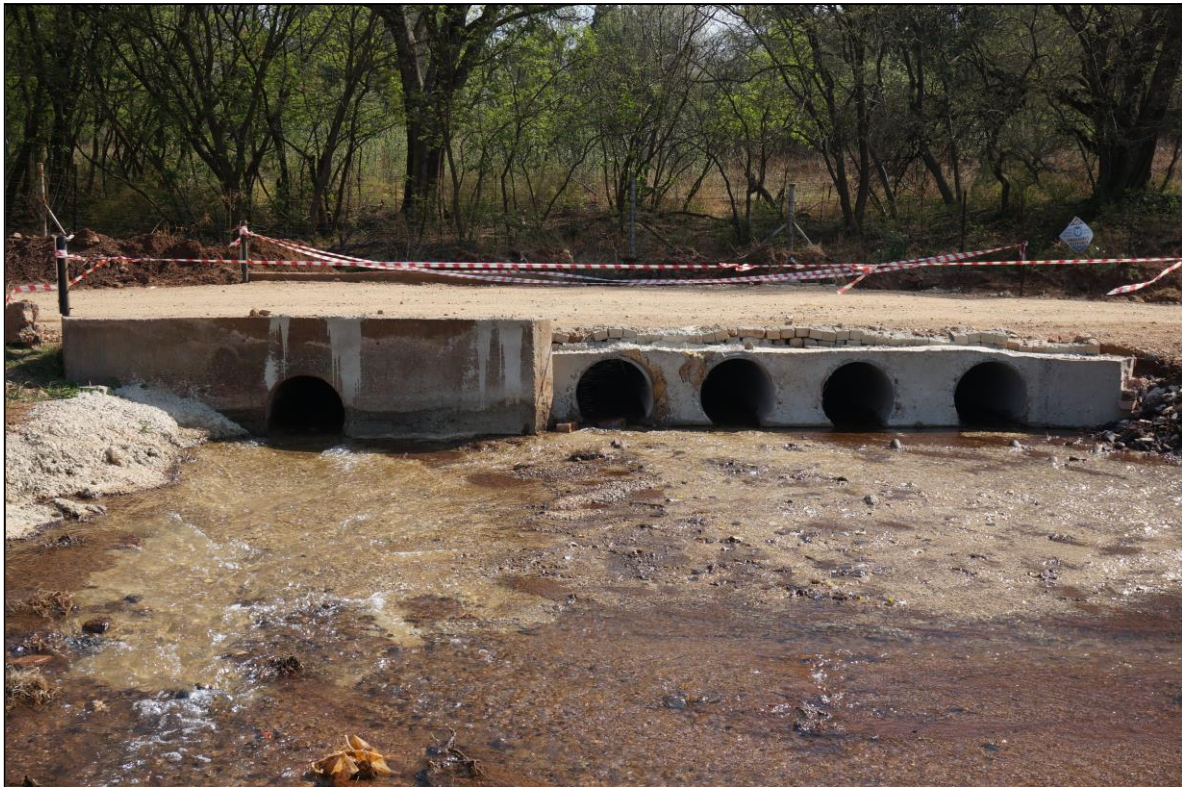
Plate 1 View of the four new culverts constructed at station MRd to accommodate high discharge conditions in the Riet Spruit arising from uncontrolled mine water discharges via the Tweelopie Spruit; the original culvert is at far left of view (photo Phil Hobbs, date 26/09/2014)
