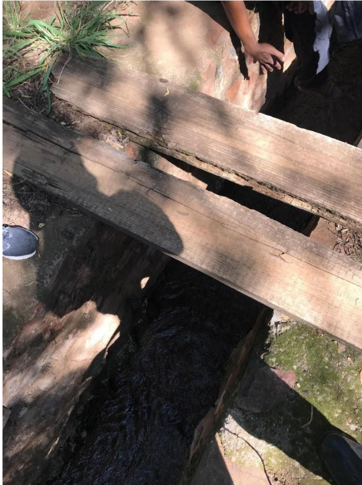
Figure 26 The concrete furrow where water from the Broederstroom spring collects as it flows downstream
