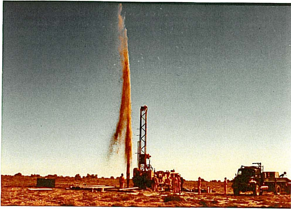
PLATE 12: Significant interconnection between two neighbouring boreholes at site 3 after blasting, as evidenced by this attempted 'blow test'
