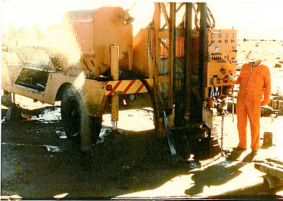
PLATE 13: Water ejected from G34350 (Left) while 'blowing' G34348. Boreholes are 1,75 m apart
