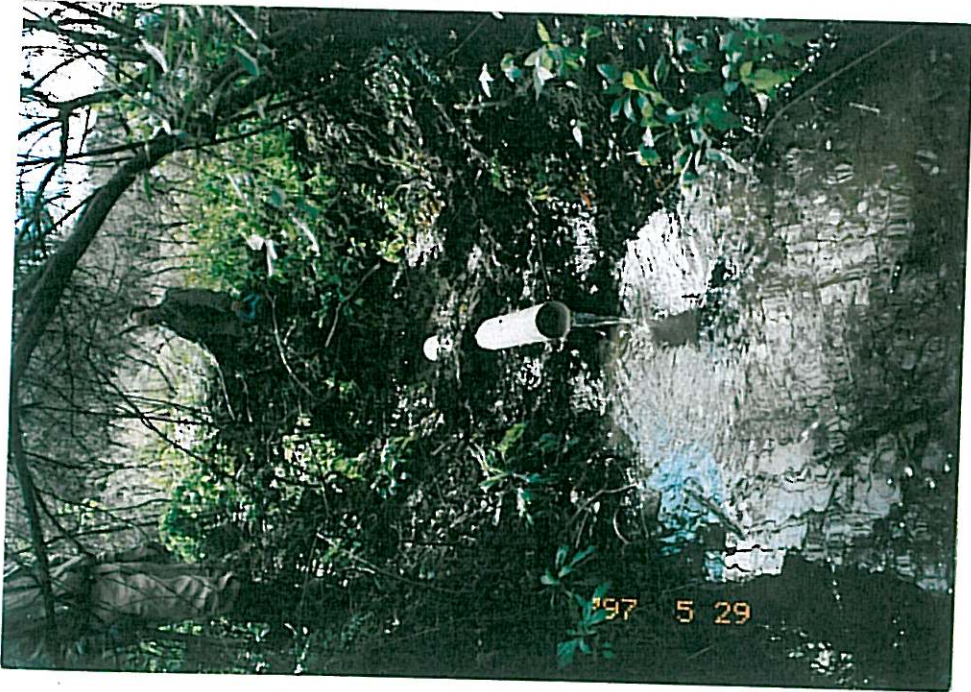
Discharge point at Spring No 3.
