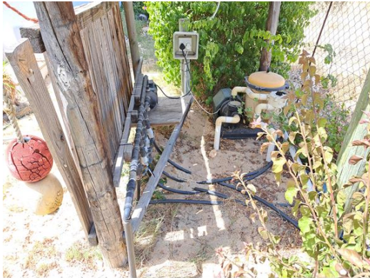
(a) Well point infrastructure
