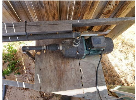
(b) 1.13kw well point pump
