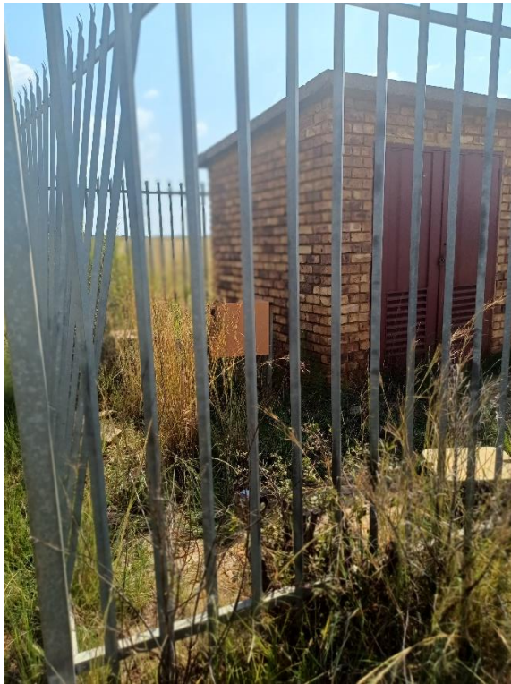
Photo 4: View of damaged palisade
