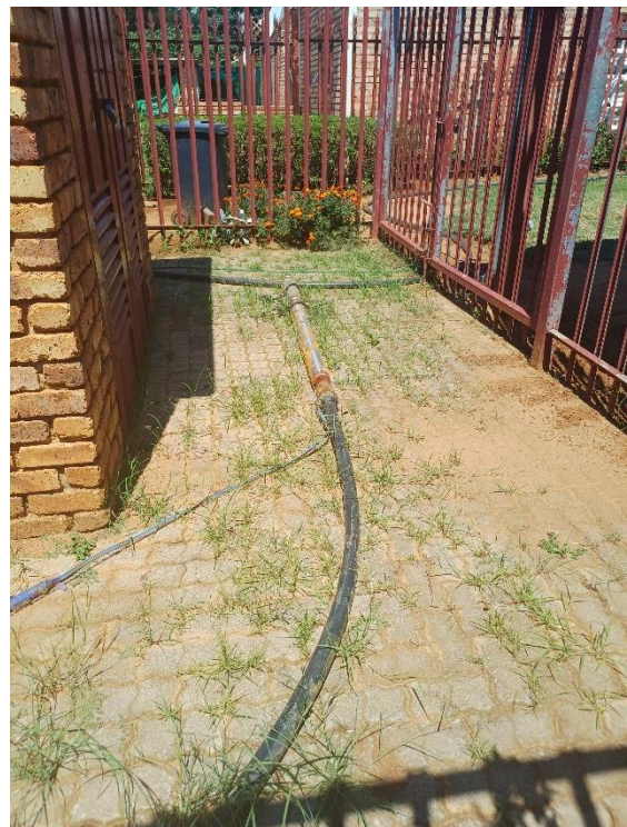
Photo 3: View of 5.5 Kw pump at BH1
