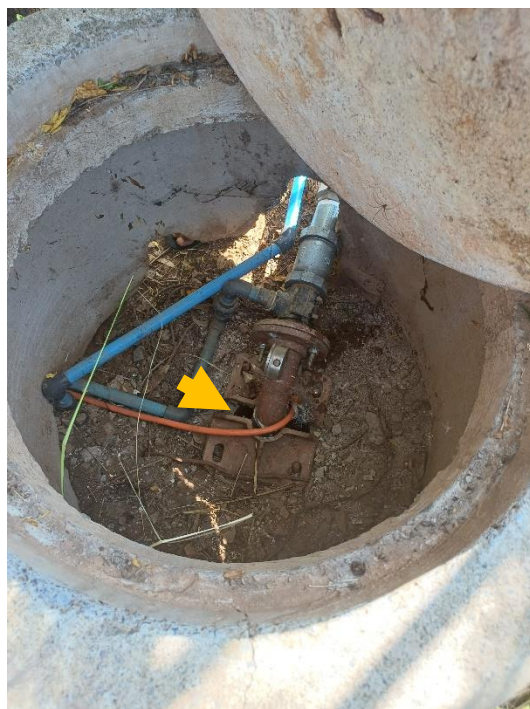
Photo 7: View of the submersible pump
