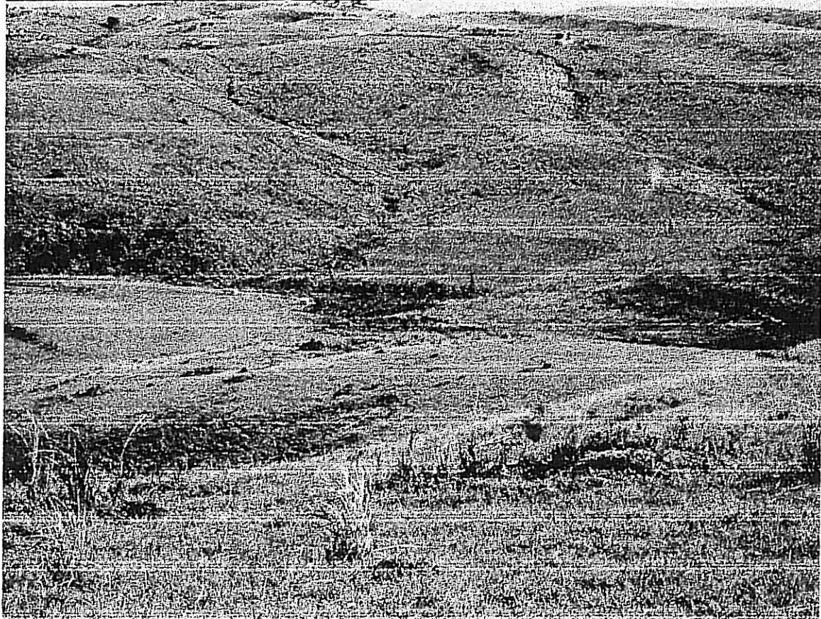
PHOTOGRAPHS 4&5: Access road works completed by local residents in area 2 is depicted in CENTANE WATER SUPPLY PROJECT – GEOHYDROLOGICAL INVESTIGATION 13
