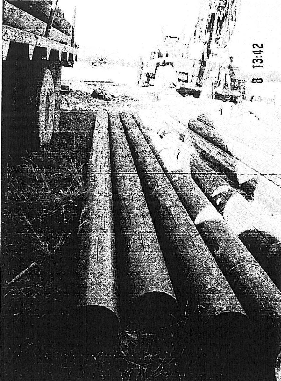
PHOTOGRAPH 7: Plasma slotted casing together with gravel packs were utilised on all boreholes with yields >5l/s or where difficult geological conditions were encountered.
