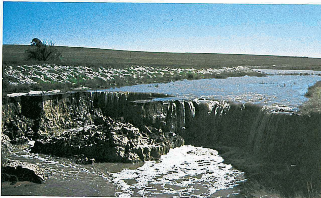
PLATE 11: An example of spillway failure
