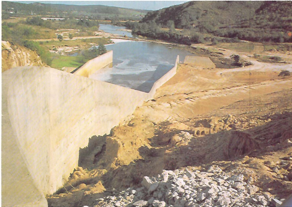
Fig. 6.2 Loerie Dam. Damage to earth embankment
