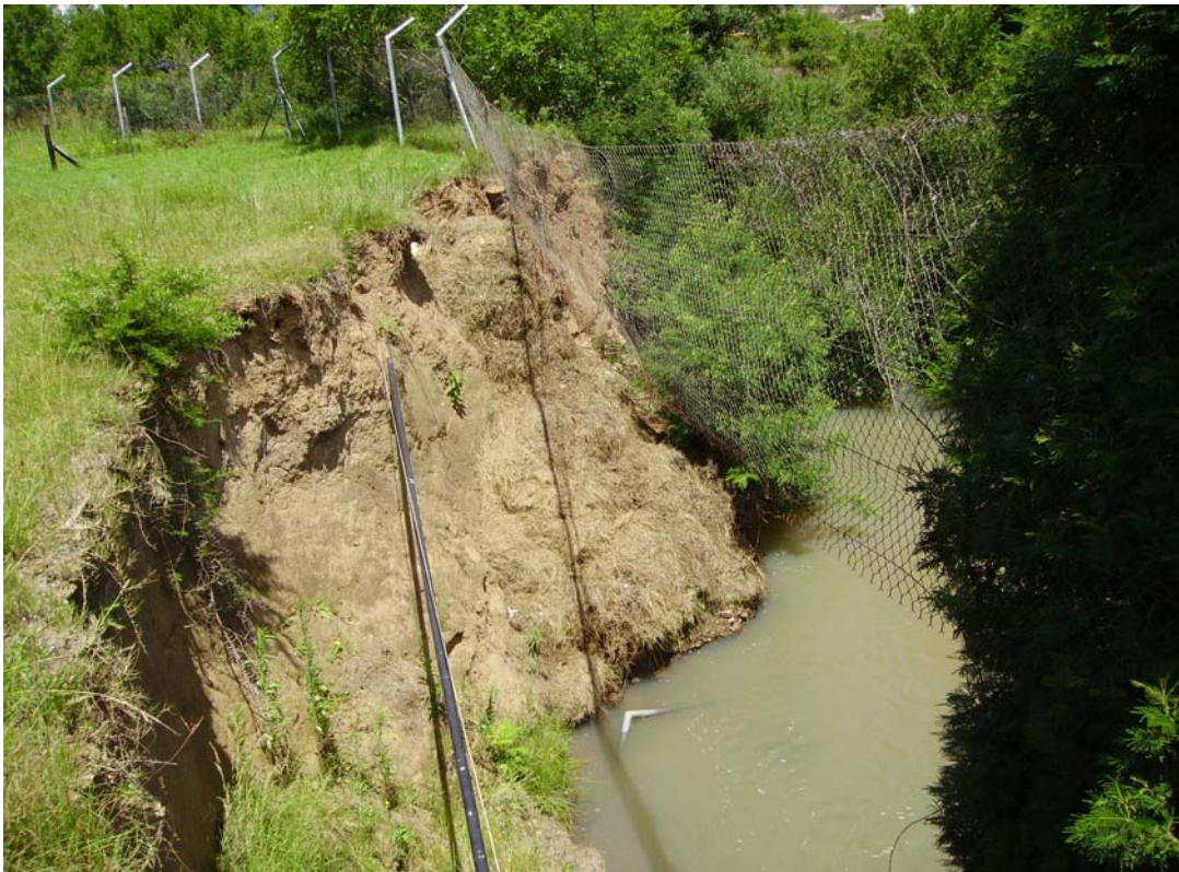
Figure 3. Badly eroded Keiskamma river banks just next to S.S Gida Hospital. The erosion is so bad that a substantial mass of S.S Gida land has been lost, leaving exposed
