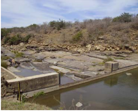
Fig 2. No water flowing over the weir wall at Mgqakhwebe.
