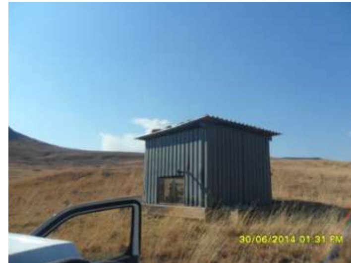
Water pump at coordinates 31 08.8654S 28 66.0927E
