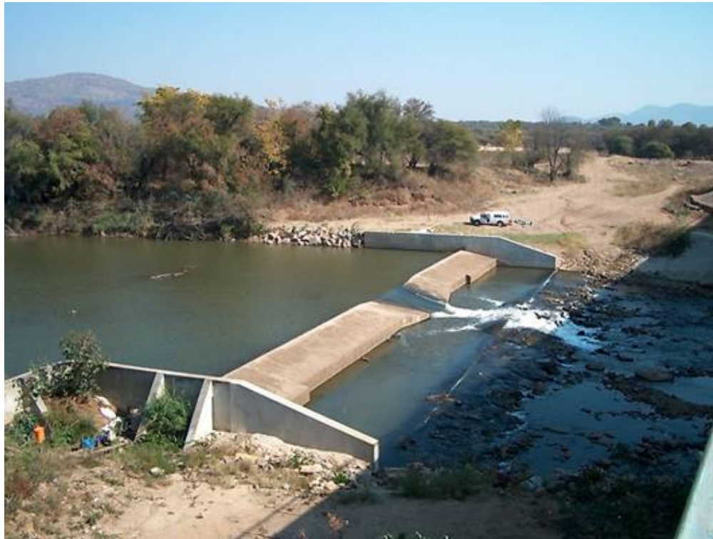
Figure 12: Flow Gauging weir in the Crocodile River at Nooitgedacht
